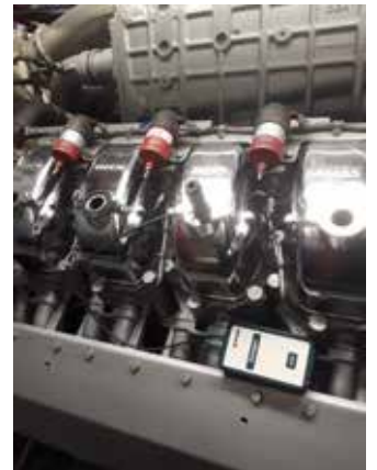
Compri installed on a power plant MTU 4000 (Powertec 1160) 4-stroke gas engine
