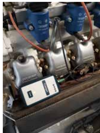
Compri installed on a power plant MAN E2842 Le312 4-stroke gas engine
